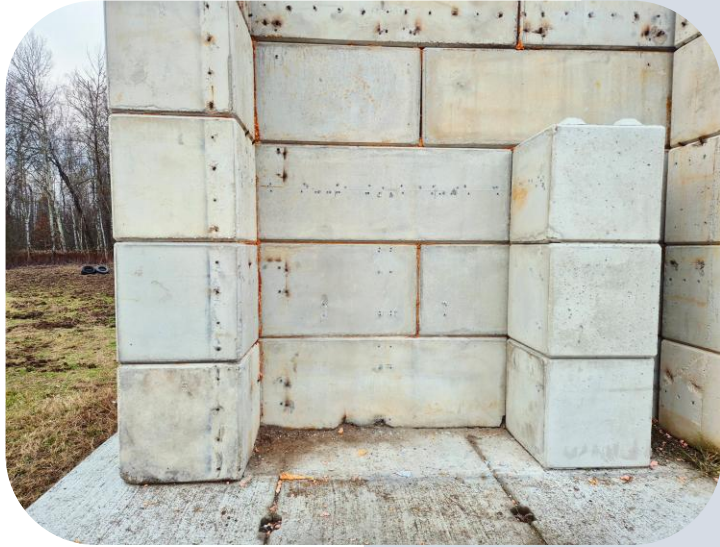
The wall before the explosion
